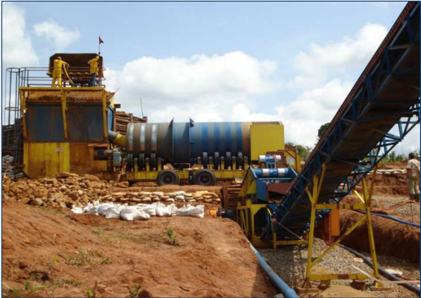
Wet feeder, scrubber and de-watering screen
